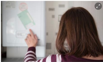
This trial boiler on prescription scheme in Sunderland was seen to make a 'massive' difference to people's lives, raising temperatures by 3C and saving £30 a month. Photograph: Gentoo
